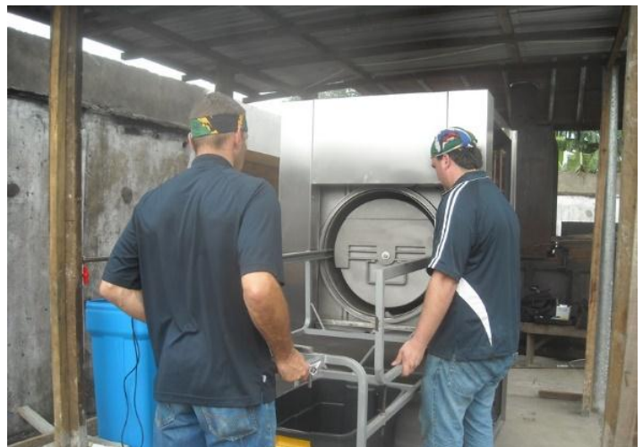
South African technical consultants installing the autoclave at Redemption Hospital, Monrovia. Credit: UNDP/ Sam Zota, 2 Sept 2015.
